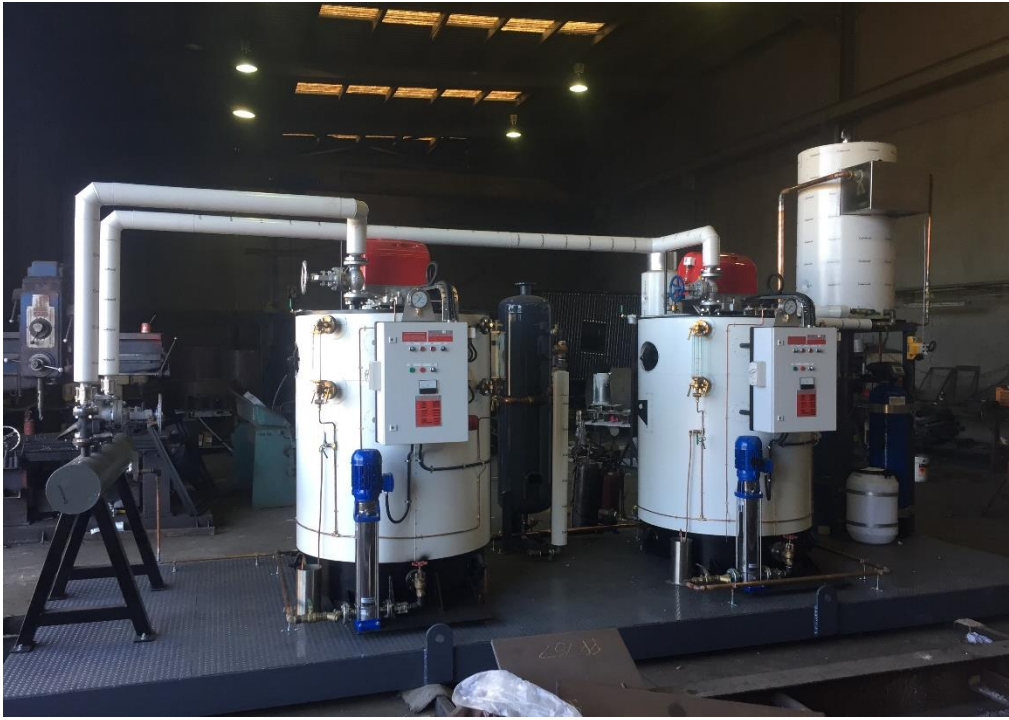
Figure 3- Image of 2 x 500 KW tandem boilers
