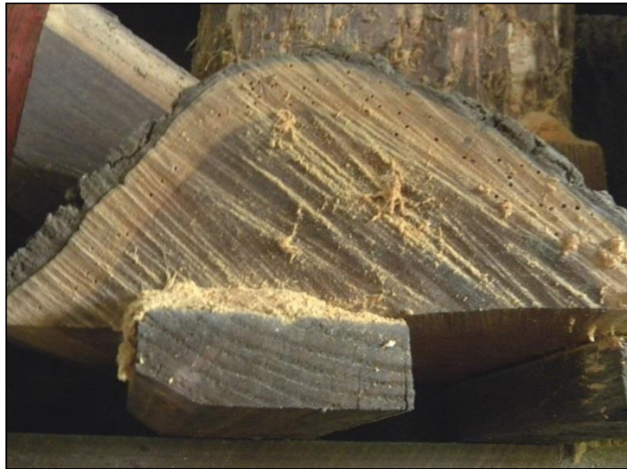
Image 4. Signs of a previous lyctid beetle infestation (borer holes and powdery frass) in a timber storage area at the DAF Salisbury Research Facility.
