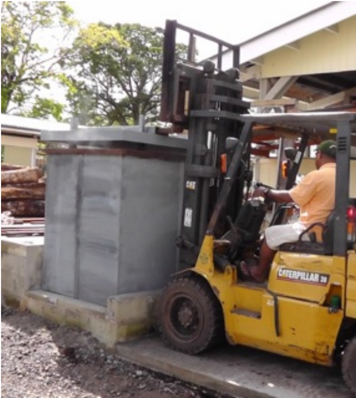
Gas-fired hot water bath: TUD Suva Experimental volume unit only
